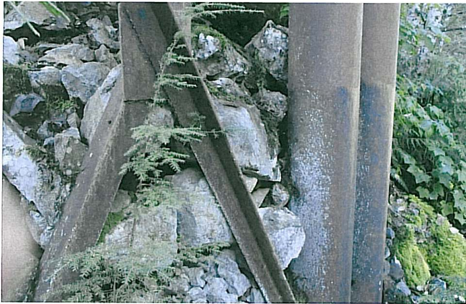
CK-2230 Pier 2 rocks at bottom
